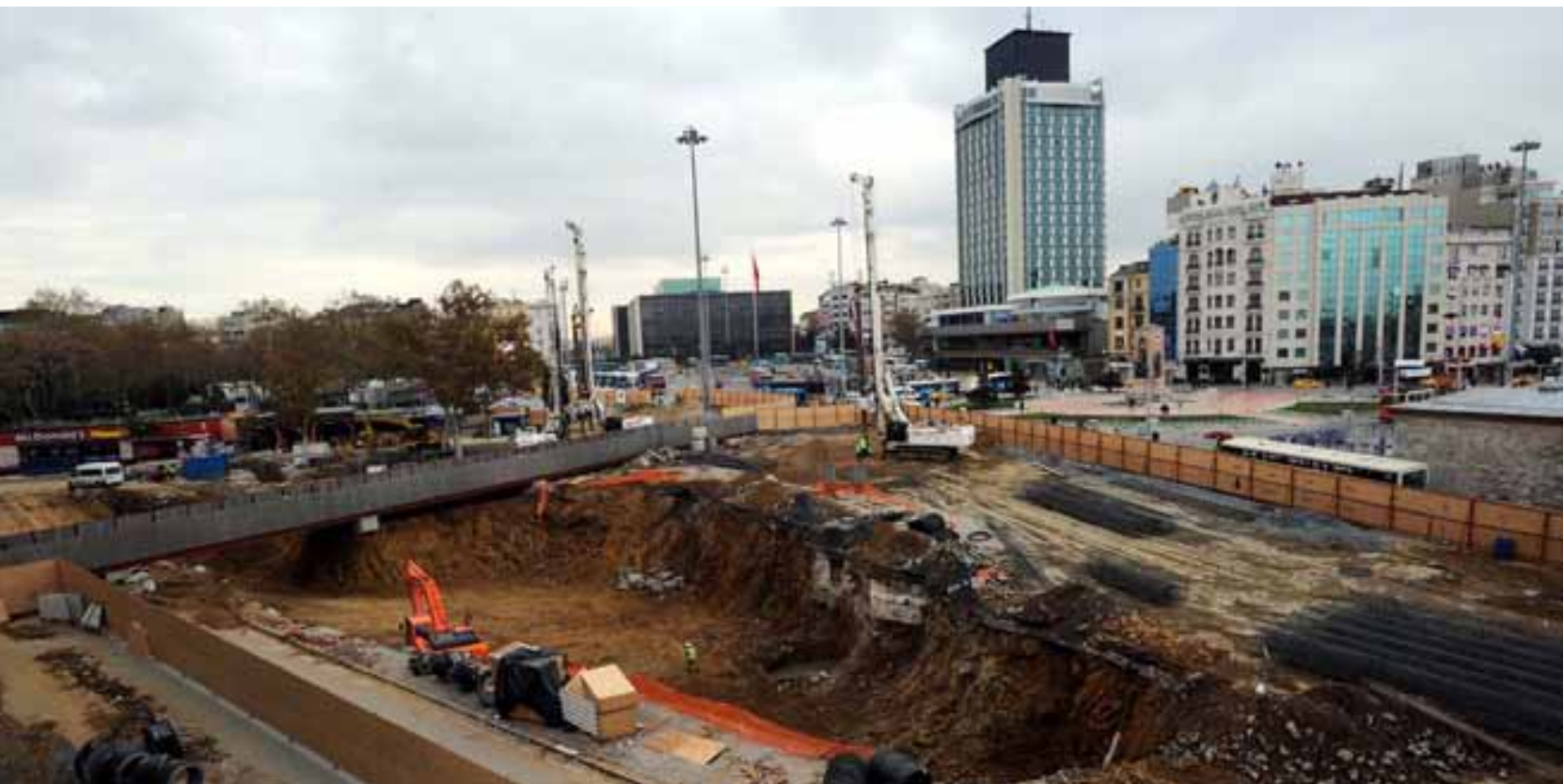
Current view of the Taksim Square where tunnel diggings started a few months ago.
